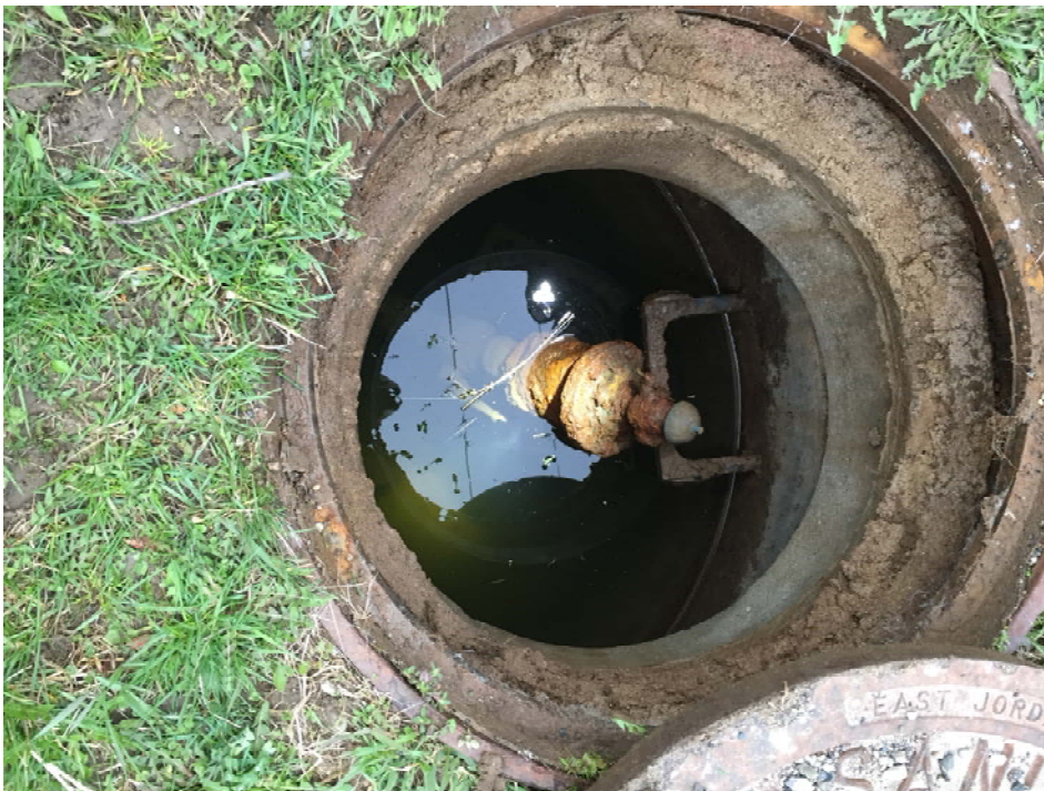
Figure 2 – Air release manhole on Boettner Road
