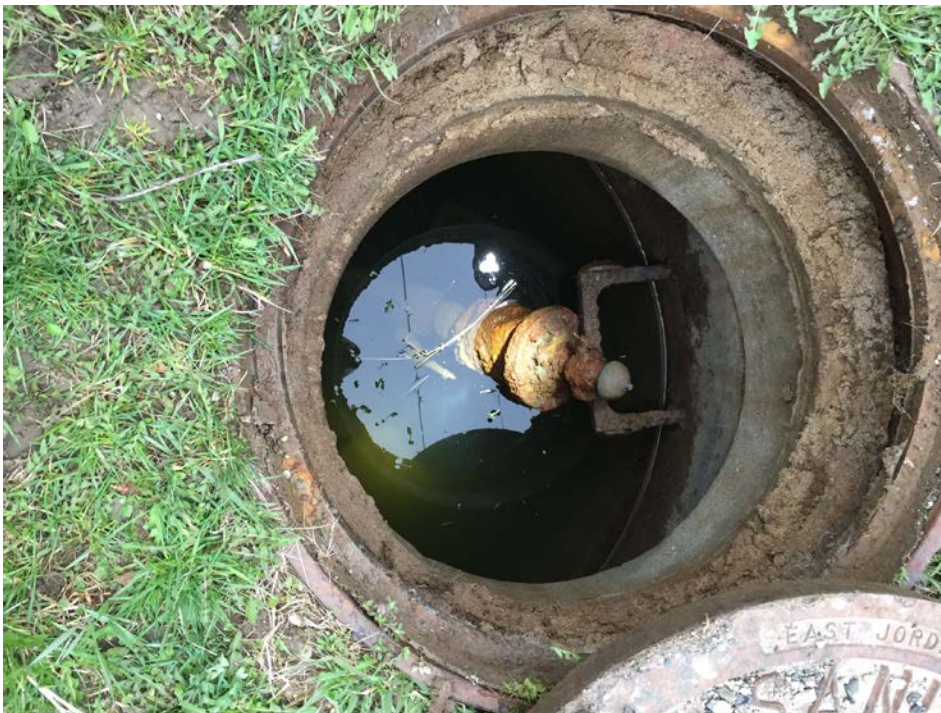
Figure 2 – Air release manhole on Boettner Road
